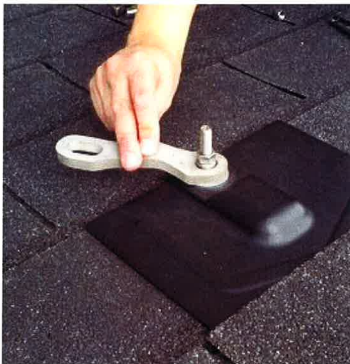
Photo 4: Final assembly showing flashing installed and swivel lug attached ready to attach body harness lanyard.
