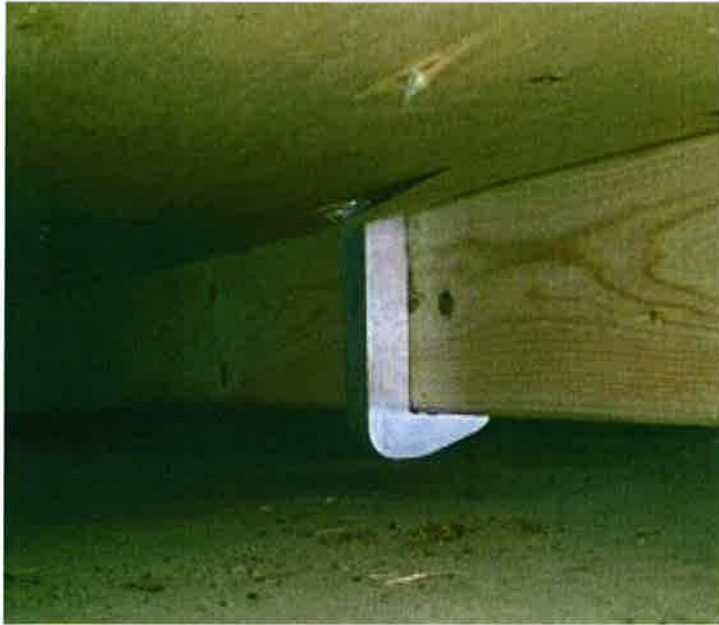
Photo 1: “J-hook” installed under roof rafter (or truss chord) through hole drilled in sheathing.
