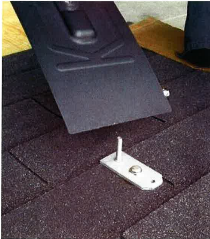
Photo 3: Top of roof showing upper plate with flashing ready to install by sliding upper edge of flashing under shingle tabs above the hole drilled for the "J-hook".
